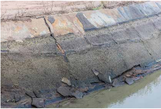
Above: This photo shows the state of the irrigation channels before the channel works were undertaken. In several locations, the old concrete was cracked and in a bad state of disrepair, leaking water.
