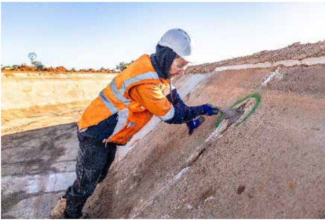
Above: As part of the works, the channels were cleaned and repaired. In some areas, where the concrete was in very poor condition, the existing concrete was removed and new concrete installed. Once the channel was repaired, new heavy duty reinforced liner was installed to prevent seepage and increase the efficiency of water delivery.
