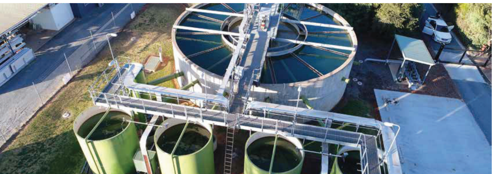
Robinvale Water Treatment Plant
