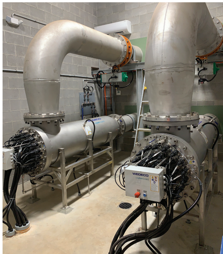
Ultraviolet (UV) disinfection infrastructure
