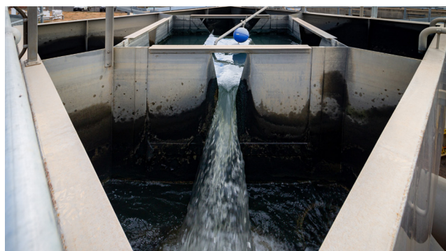
Water Treatment Plant in-flow splitter box
