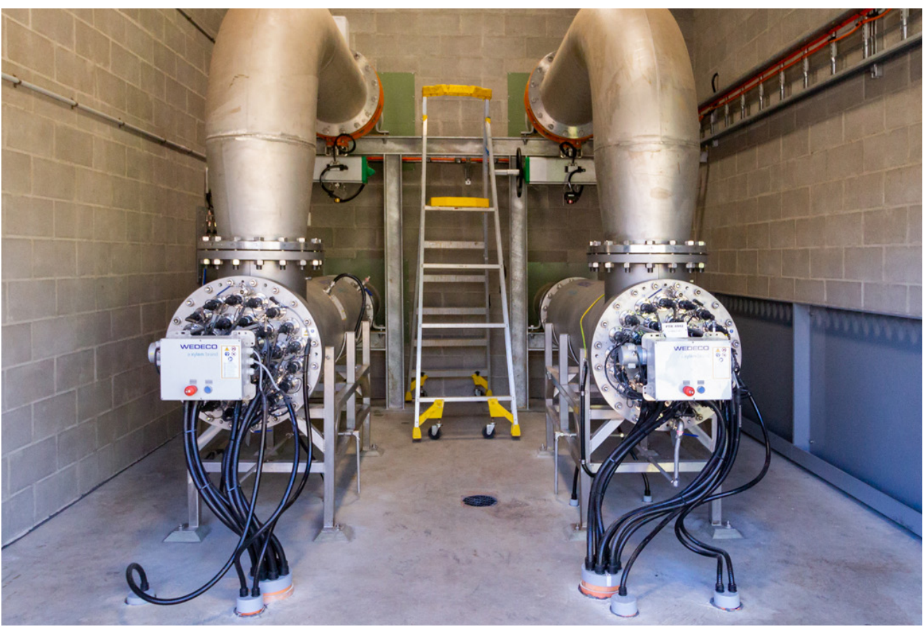
UV Disinfection, Red Cliffs Water Treatment Plant
