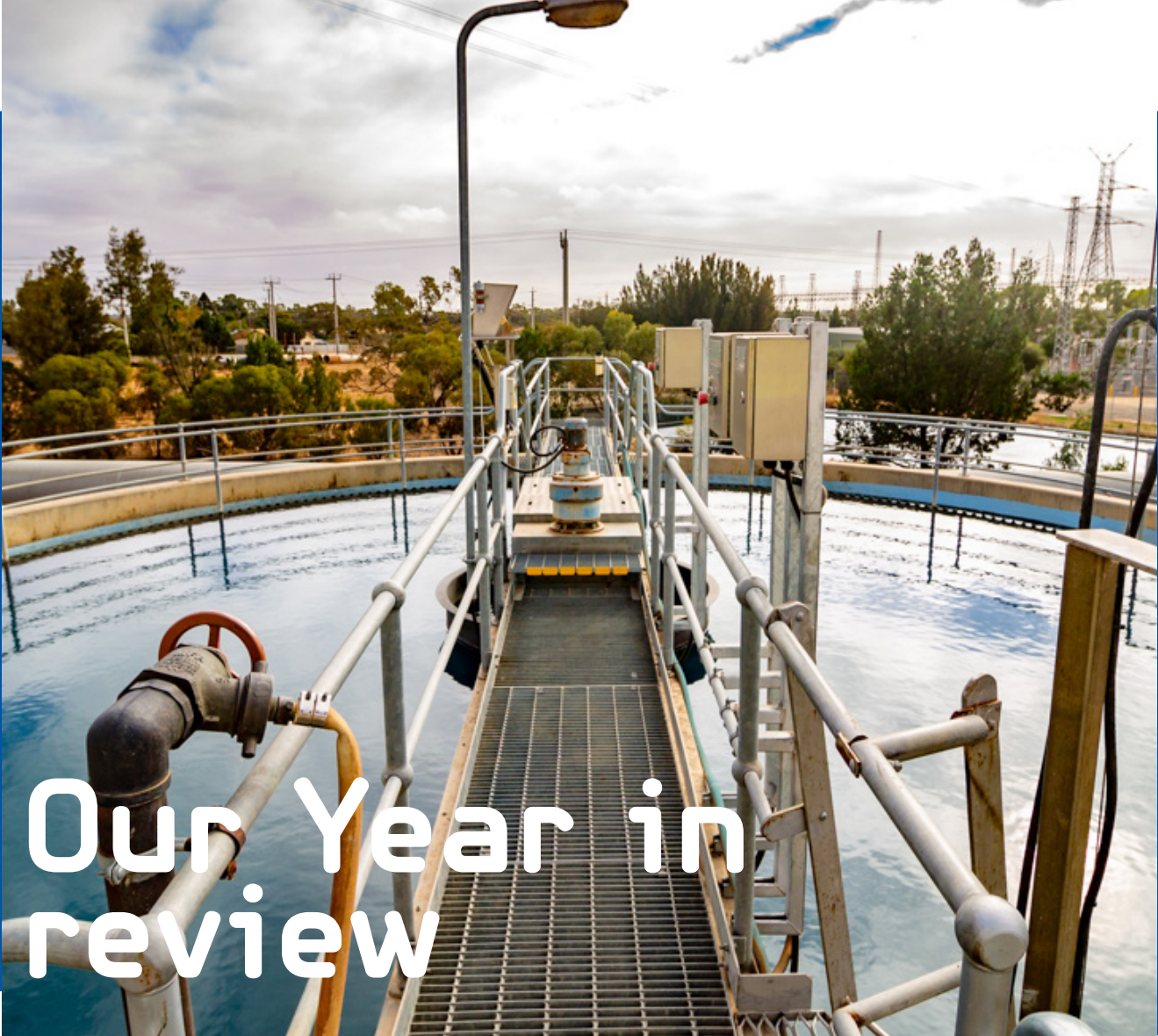
Red Cliffs Water Treatment Plant
