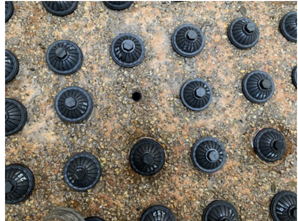
Figure 3 - Missing nozzle from Robinvale WTP Filter #1
