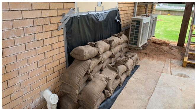
Sandbagging at Kerang WTP as part of the IMT planning phase to protect the community drinking water supply.
