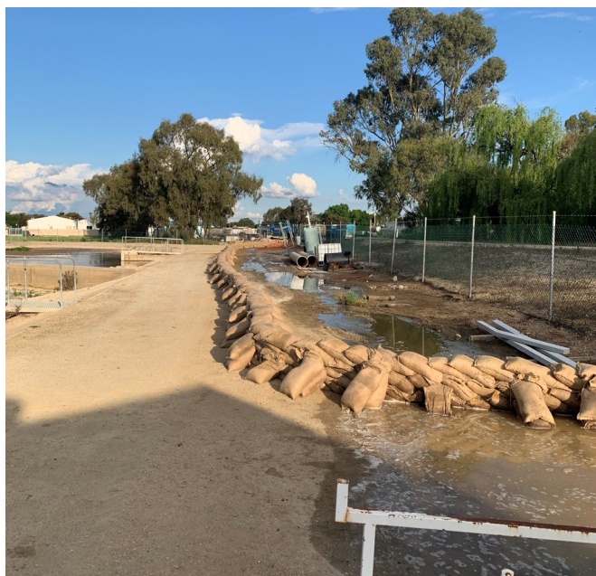
Community sandbagging efforts at Kerang WTP to control a leak in the levee alongside the Loddon River.
