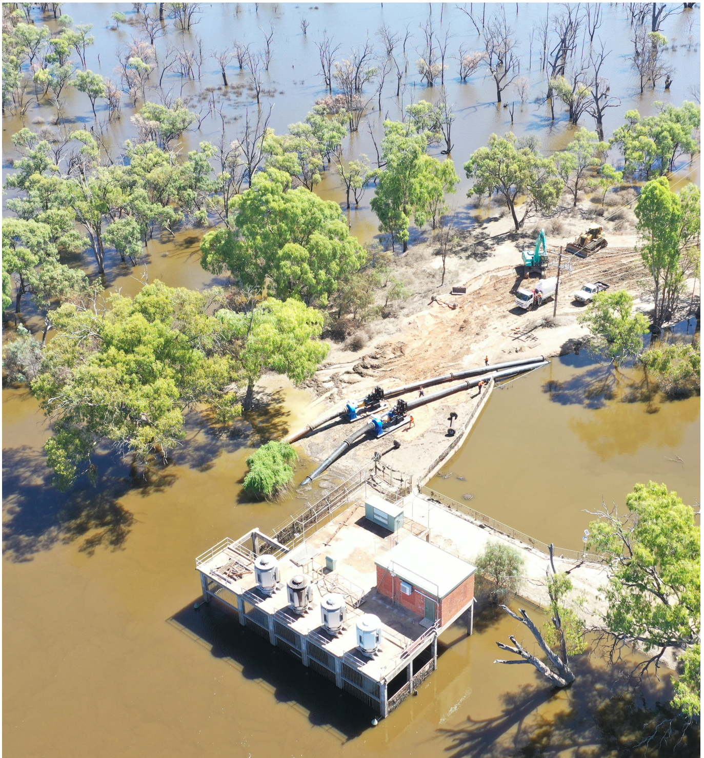
Psyche Irrigation pump station surrounded by floodwater, with emergency pumps in situ following the disconnection of electricity to the pump station.
