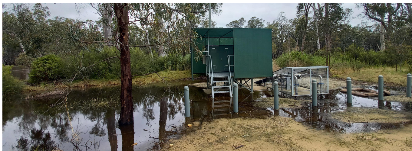
Murrabit WTP raw water pumps surrounded by floodwater.
